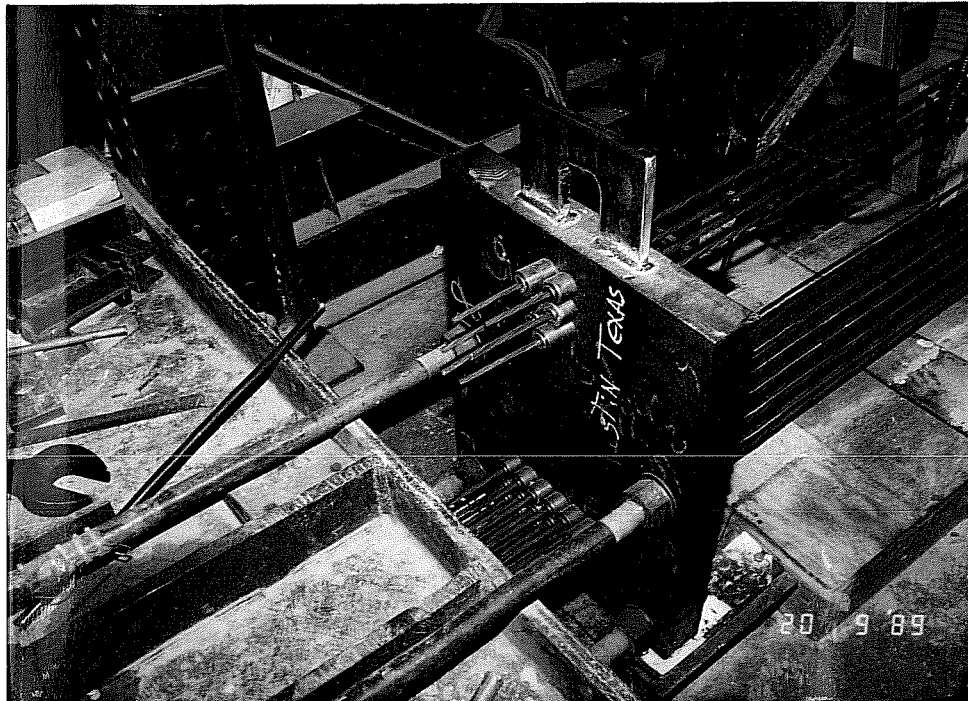
Figure 3.21 End Plate of Prestressing Bed
